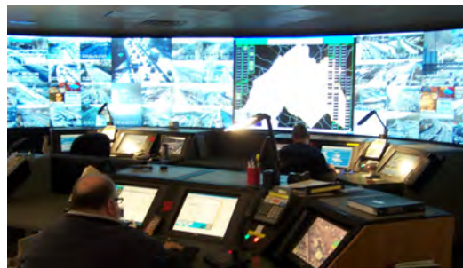
Traffic control center at the PennDOT District 6 offices.
