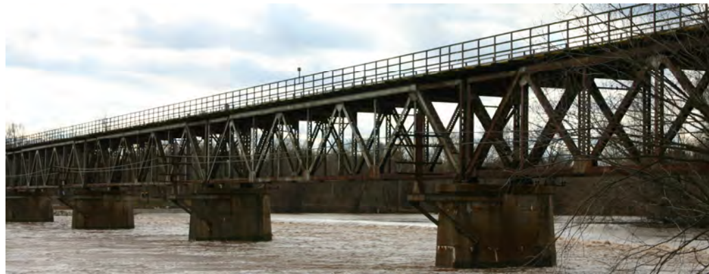
Funding has allowed for badly needed repairs to be made to the Bridgeport Viaduct; without these repairs, service on the Norristown High Speed Line into Norristown could have been severely impacted.
