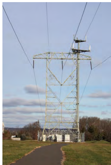
Wireless communications antennas may be hidden within structures (as in the church steeple on the right), placed in plain view, or put on existing structures like the power line on the left.
